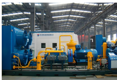
Station de compression de gaz
